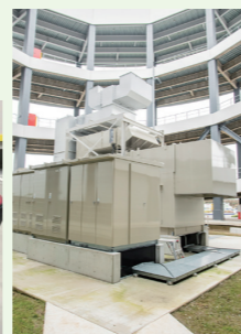
In-house power generation facilities
