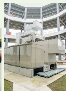
In-house power generation facilities
